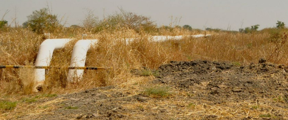
Oil pipeline that runs from Bentiu to Yida, South Sudan. Photo by Shannon Orcutt
